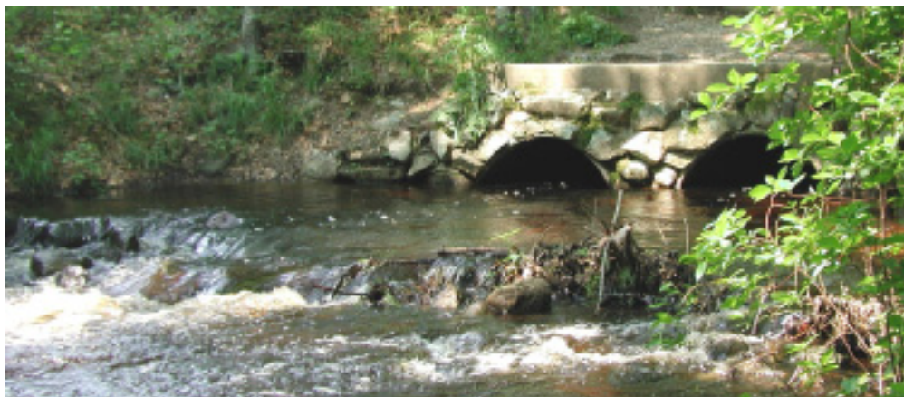
Stream Baffles at Rochester Fish Hatchery
