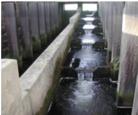
Upper (weir-pool) Section of Tihonet Pond Ladder
