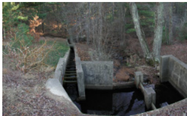
Lower (Denil) section of Tihonet Pond Ladder
