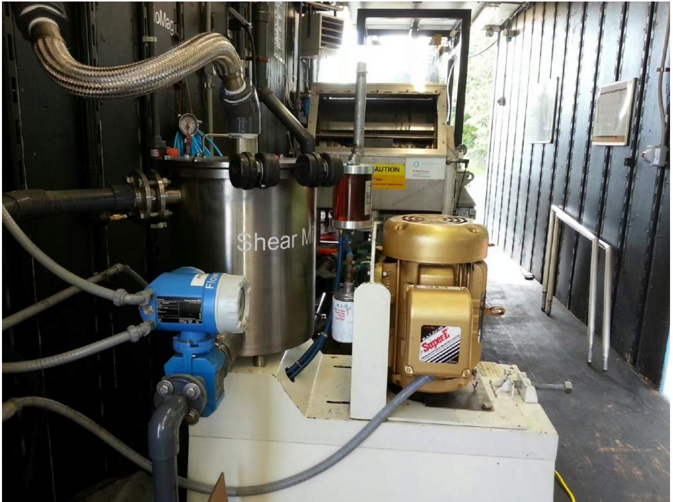
Figure 6 - Shear Mill (Foreground) and Magnetic Recovery Drum (Background)
