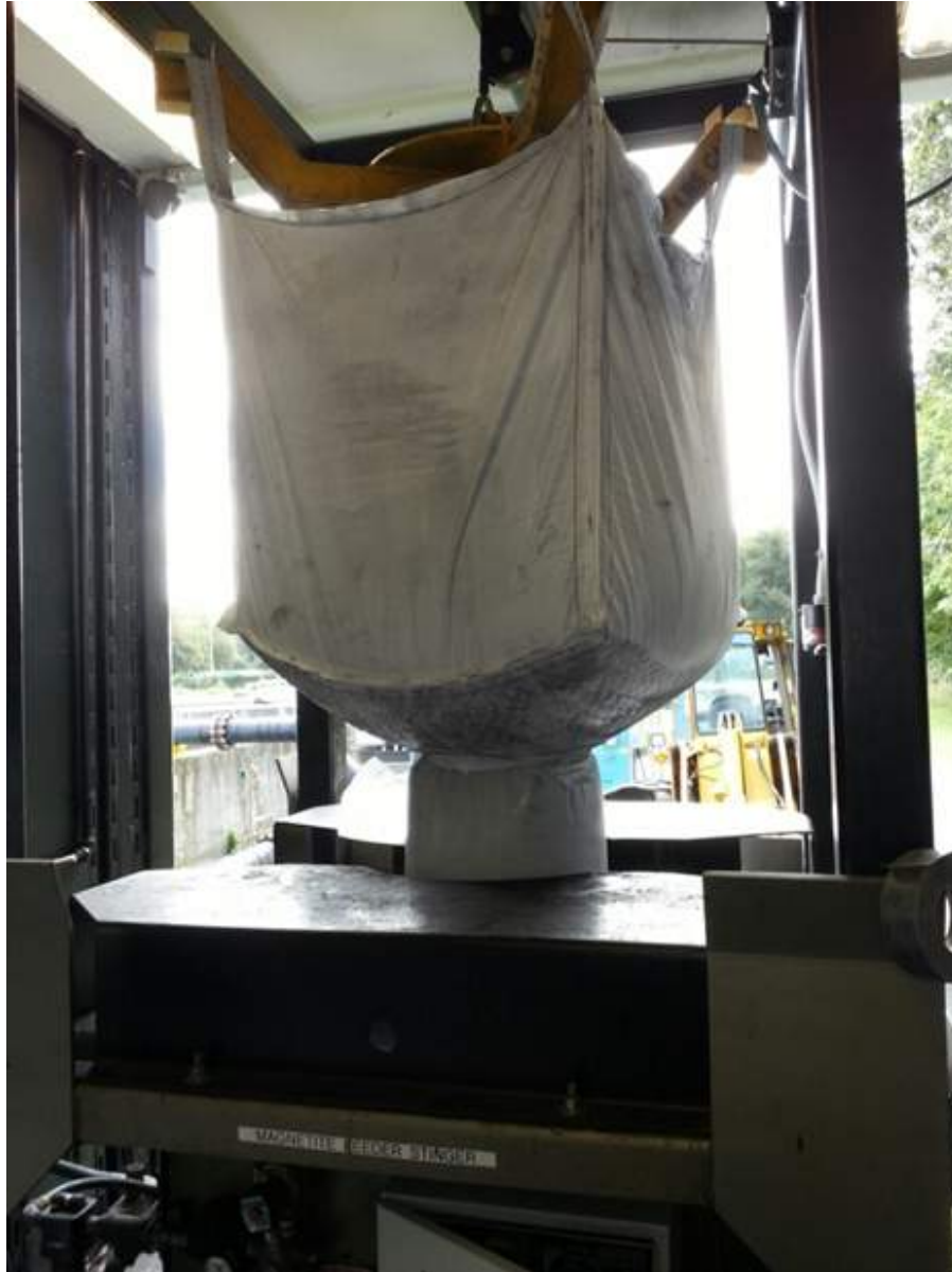
Figure 4 - Automated Magnetite Feed System
