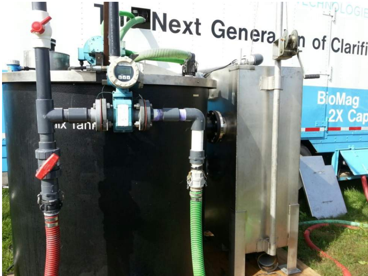
Figure 5 - Ballast Mix Tank
