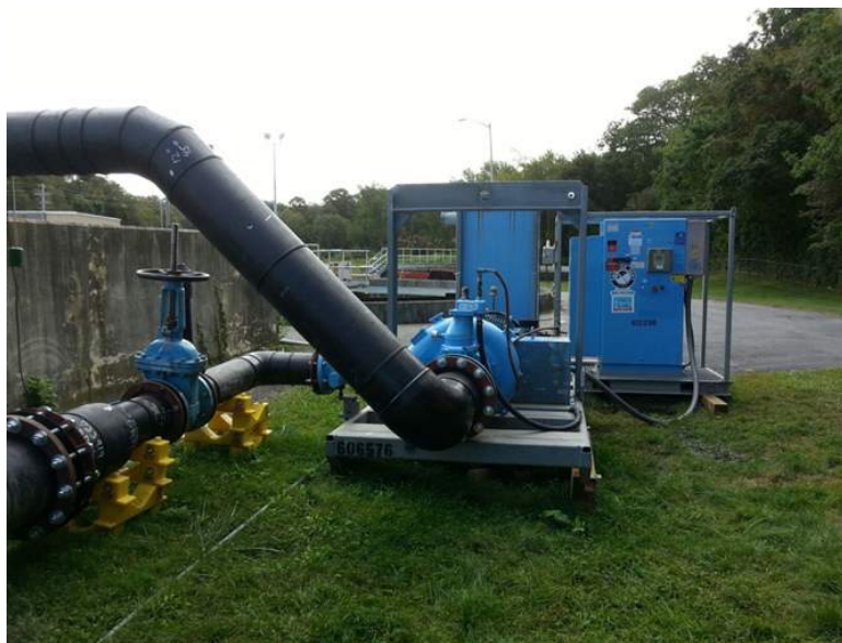
Figure 2 - Internal Recirculation Pump Rented by Town
