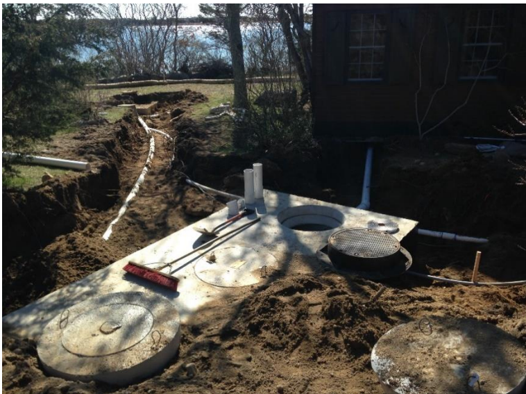
2,000 Gallon Blackwater Tank installed in parallel with an existing Title V systems at the location of Case Study BW9.
