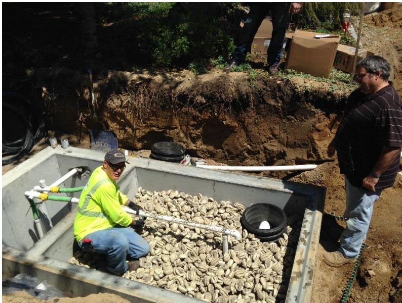
Eliminite Tank installed in parallel with an existing Title V systems at the location of Case Study EL3.
