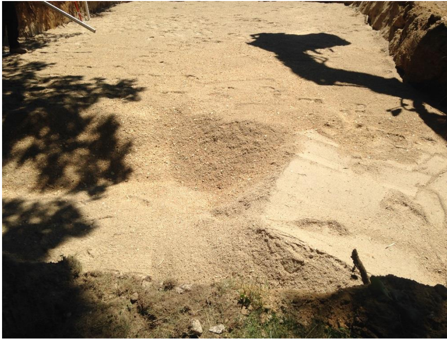
Layered STA installed as part of a full upgrade from cesspools at the location of Case Study #6.
