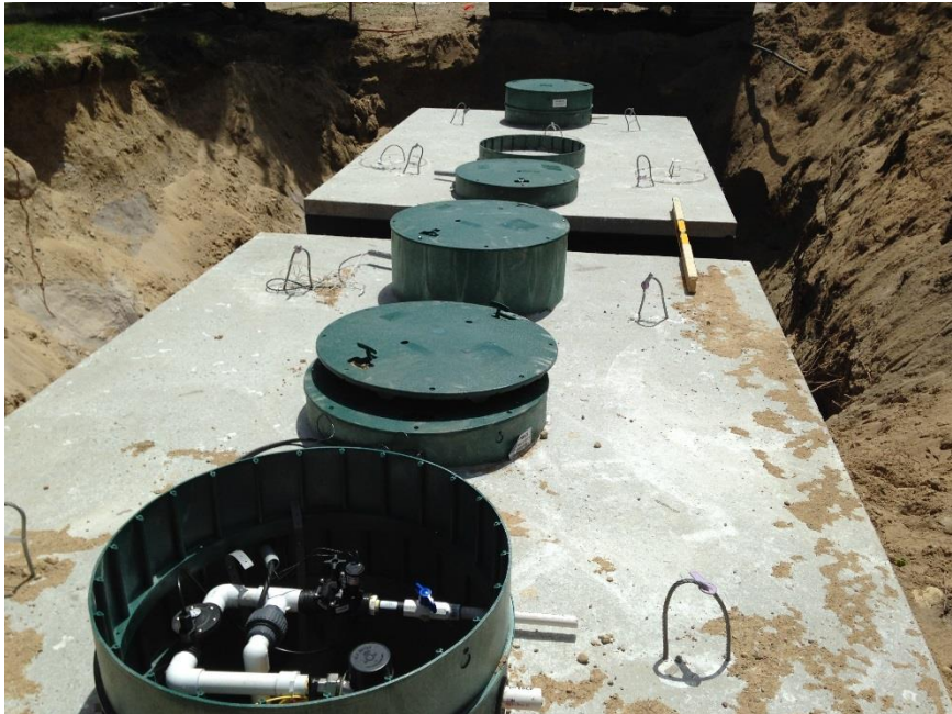
Hoot system installed as part of a full upgrade from cesspools at the location of Case Study HO2.
