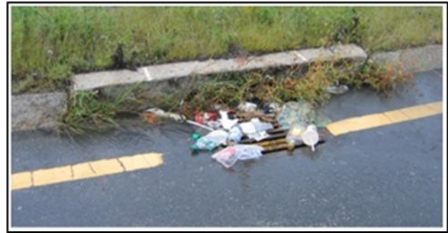
Figure 72. Litter accumulating on a storm drain grate.
